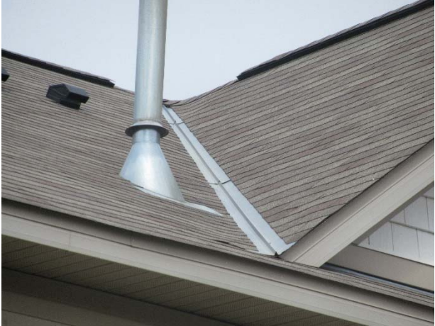
Minor sheathing deflection adjacent to valley at Bluebird Lane
