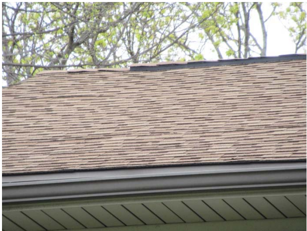
Sheathing deflection at Jackson Street
