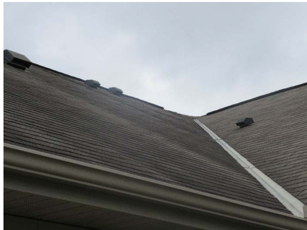
Roof sheathing deflection at Jackson Boulevard
