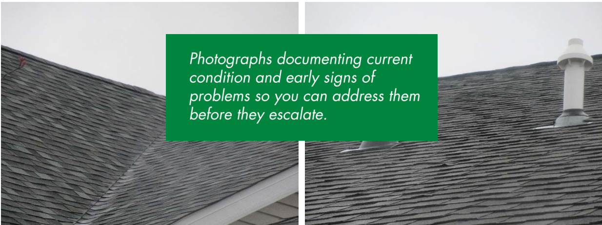
Roof shingle lift at valley
